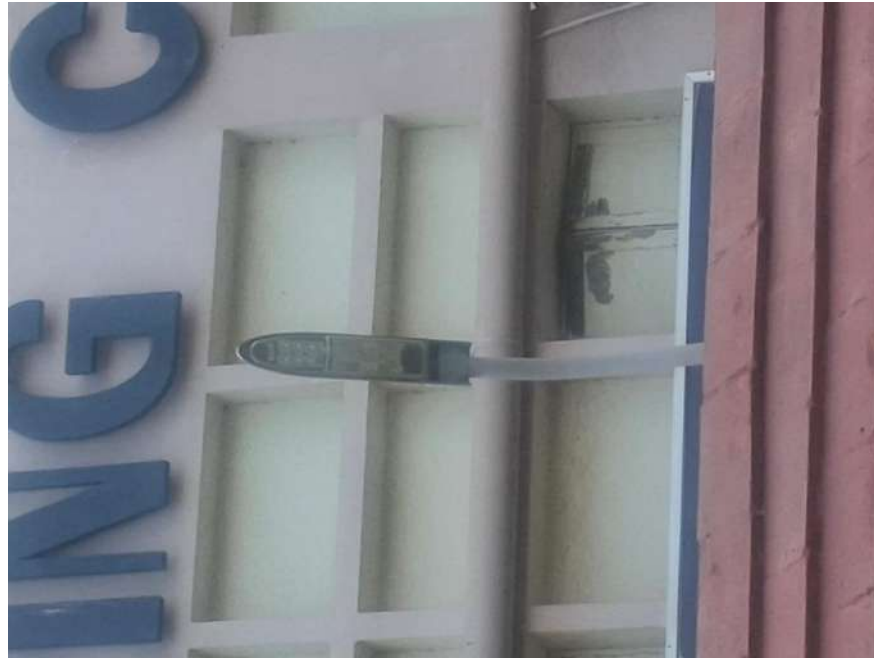
Energy-Efficient LED Lighting Installation, Main Block
