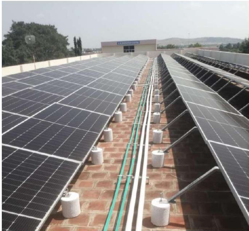
Rooftop Solar Photovoltaic Installation, National Engineering College Campus
