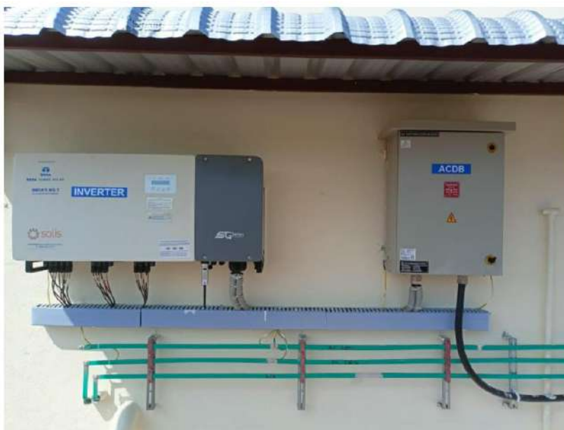
AC Distribution Board (ACDB) — Solar Power Integration
